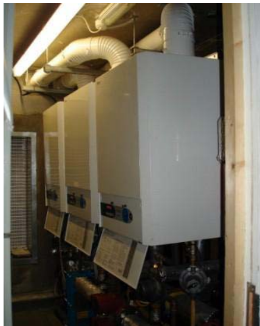
Natural Gas condensing boilers at Lagan Valley Hospital
